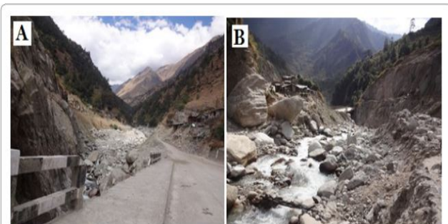
Figure 2: (a) Damaged barricading of bridge together with eroded road at Mangti area due to stream erosion by Simkhola Gad, (b) Accumulated sediments on the right bank of the Simkhola Gad.
