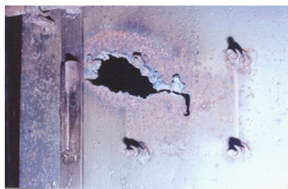
Figure 12: Gas cut marks on the strong room door.
