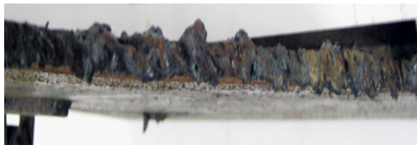
Figure 14: The gas cut tool marks on the piece of the strong room door.
