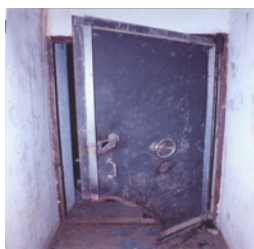
Figure 2: The damaged strong room.
